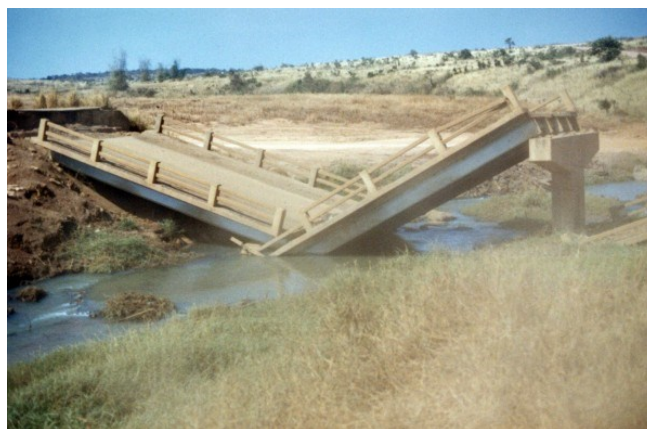
Hwy. 19 Bridge. What engineer thought it was a good idea to wave this red flag?
